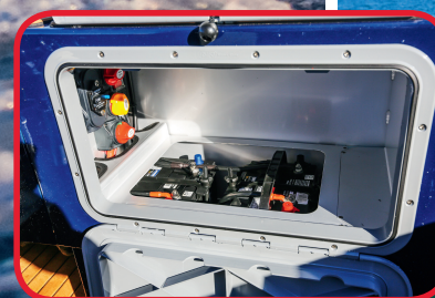
Part of the re-jigged bait station, the batteries have their own compartment with additional dry storage adjacent to the switches
